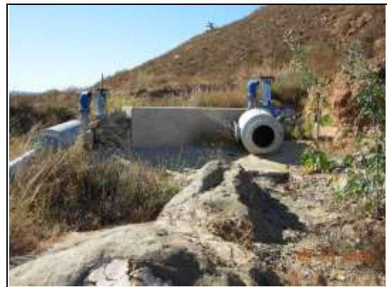
Photo 2.3: Existing outlet connection point at the dam on Portion 523.
